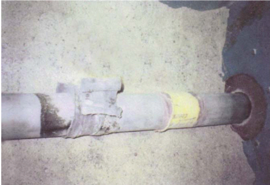
FIGURE 9 – Soil Ingress between Adhesive and Topcoat
