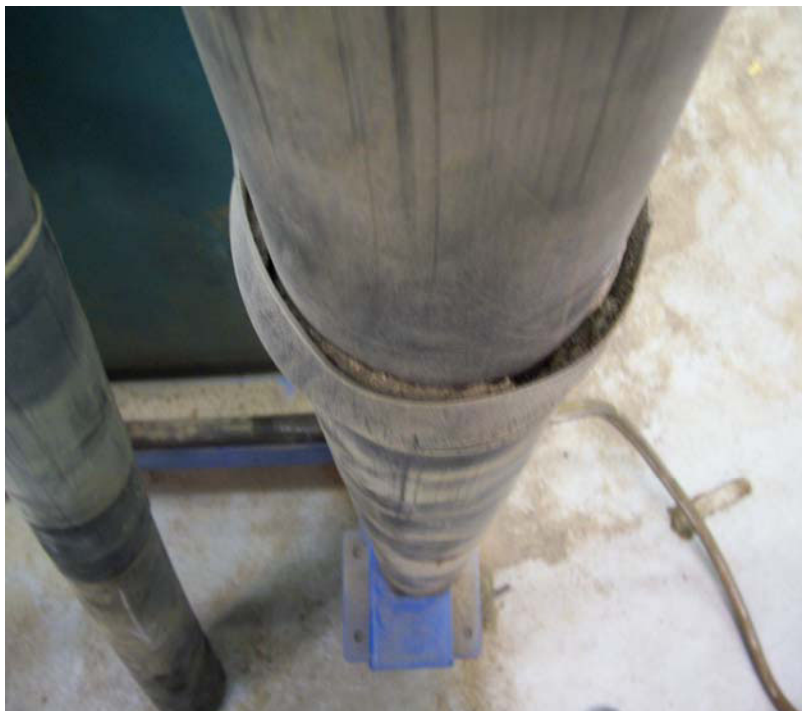
FIGURE 8 – Failure due to Soil Ingress.
