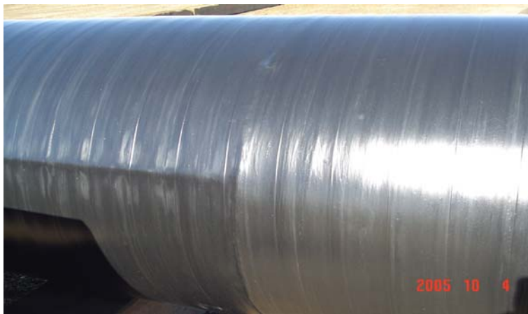
(c) Intersection of the Long Seam and the Girth Weld on Double-Jointed Pipe
